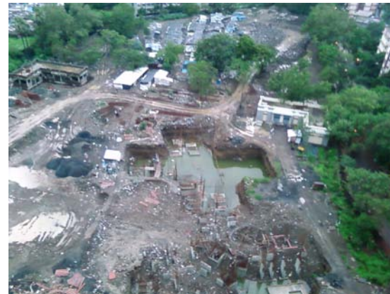
Figure 5: Construction site of CHEER tower, and behind it, the temporary labor camp built from of blue tarps and recycled sheet metal that houses workers and their families.
